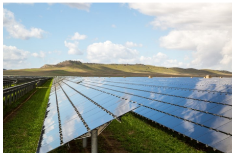
Topaz Solar Farms, San Luis Obispo, Calif. (Source: Berkshire Hathaway Energy)
